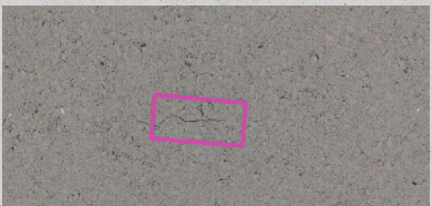
Bounding box pink: Crack
