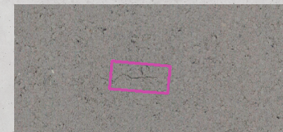
Bounding box pink: Crack
